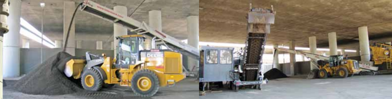
Above: Stockpiled RAP being processed as CCPR at the recycling site provided by the City of Glendale. After recycling with the engineered emulsion, the asphalt is loaded into trucks for subsequent delivery to the paving operation.
