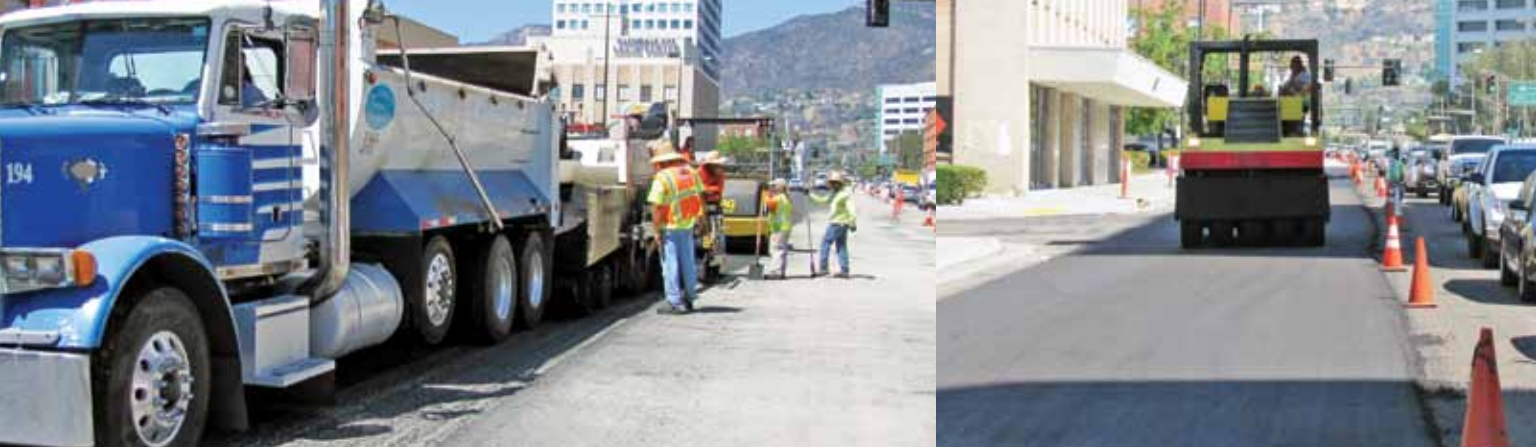
Above: Excel Paving completes the placement, paving, and rolling of CCPR asphalt. The milling was completed in seven days, while the CCPR was finished in just three shifts. Other rehabilitation methods would have required another three weeks of work, increasing the impact on the surrounding businesses and residents.
